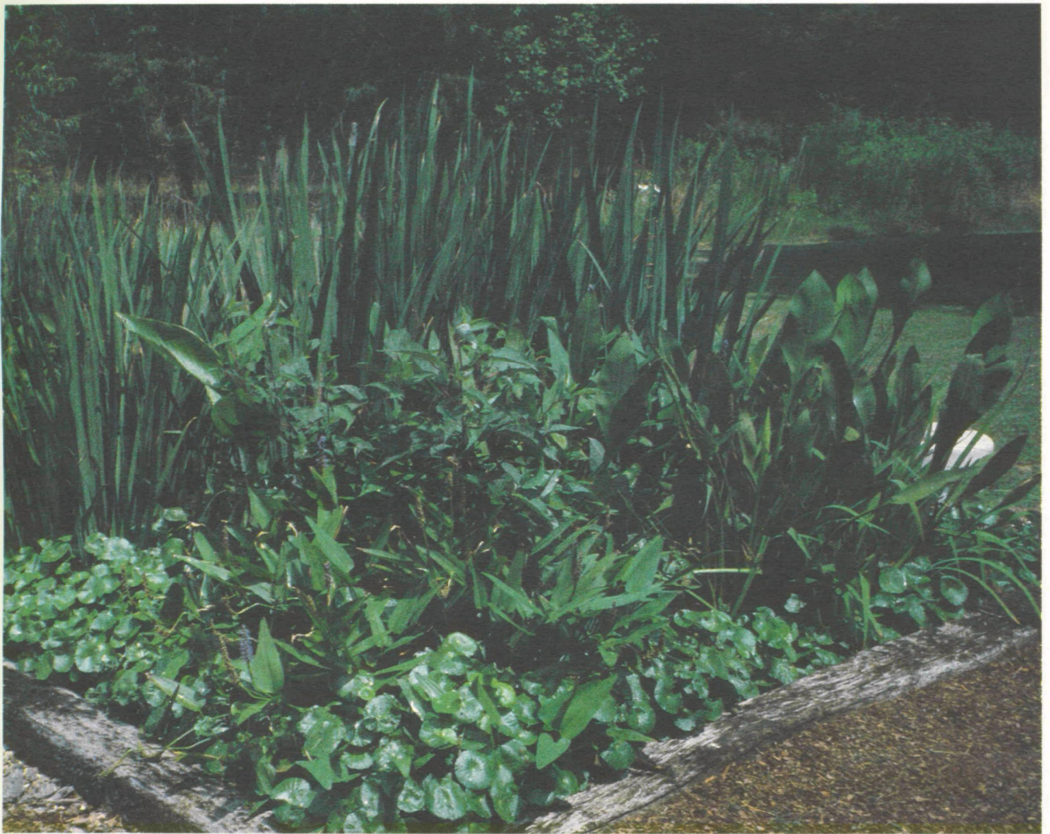
Innovative "constructed wetlands" provide homes with secondary treatment of wastewater in areas where poor soils preclude use of conventional drain fields. Tennessee Valley Authority photo.
