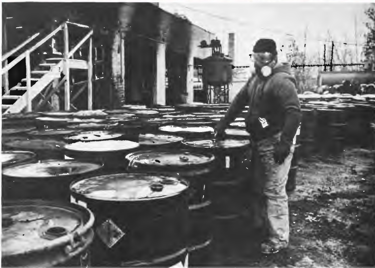
Workman preparing drums of hazardous waste for reprocessing at the Silresim site in Lowell, Mass.
