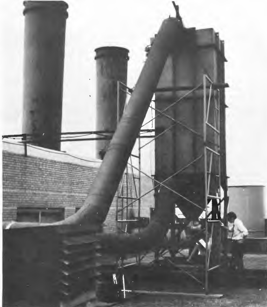
Filters inside sheet metal housing catch emissions of particles from coal-fired boilers at General Motors plant in Warren, Mich.
